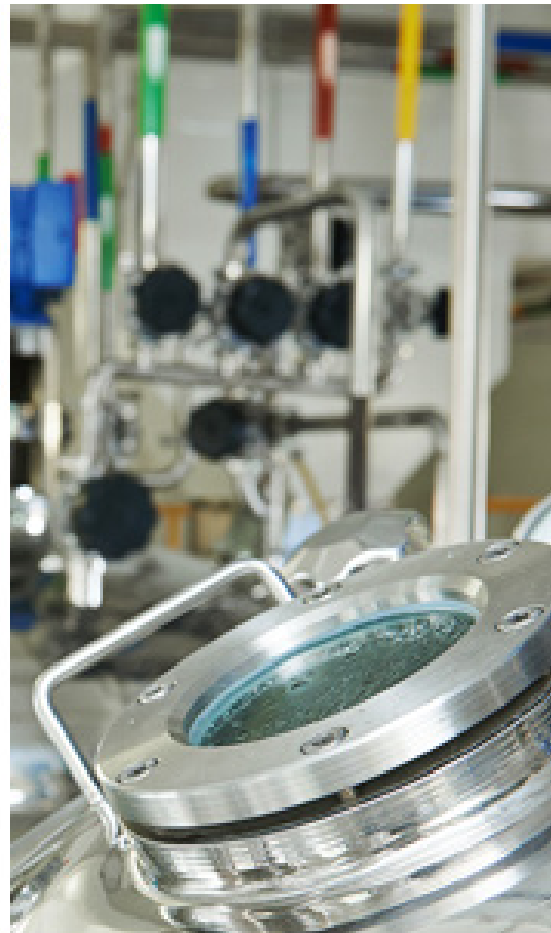
White room and chemical industries
